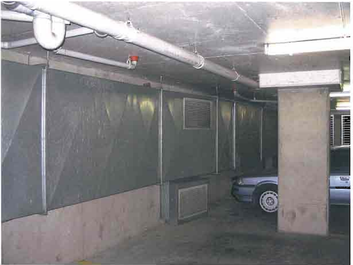
Photo No 23 Bi-Lo Carpark, air conditioning ducts
