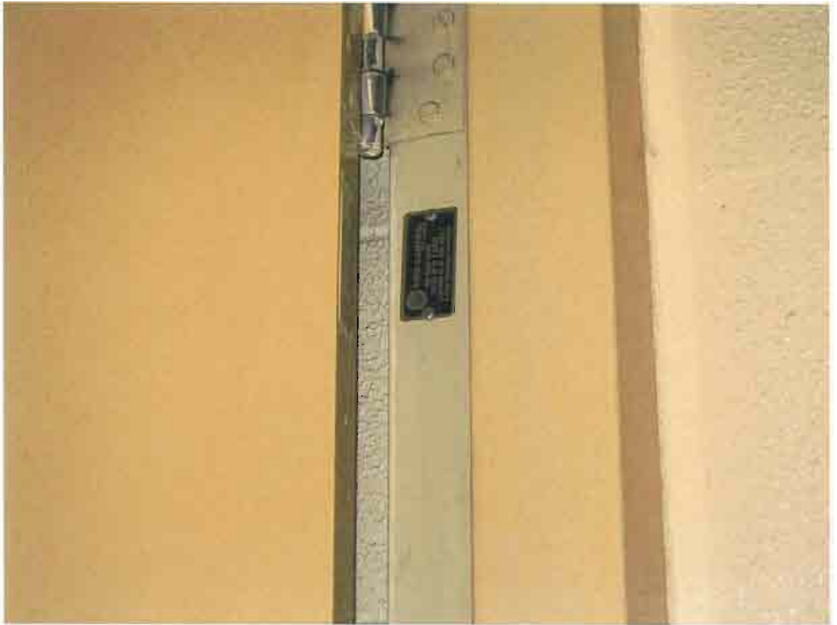
Photo No 7 1 st Floor Stair 'Fire Control' fire door tag
