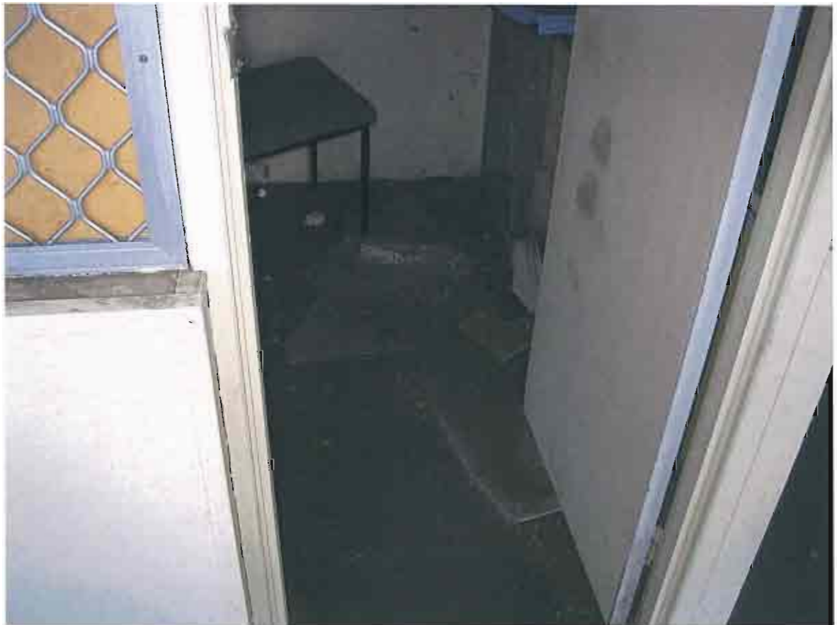
Photo No 22 Bi-Lo Carpark internal guard box – fibrous cement debris
