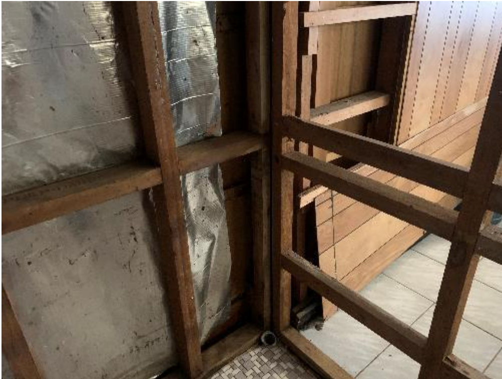
Image 5. View to the eastern and northeastern walls of the Male Toilet following the removal of asbestos cement sheet.
