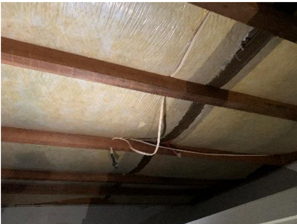
Image 6. View to the ceiling of the Female Toilet following the removal of asbestos cement sheet.
