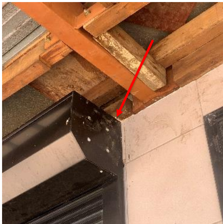
Image 2. Detail view of the asbestos cement sheet trapped between the metal roller shutters and timber framework. This ACM should be removed as demolition works progress.
