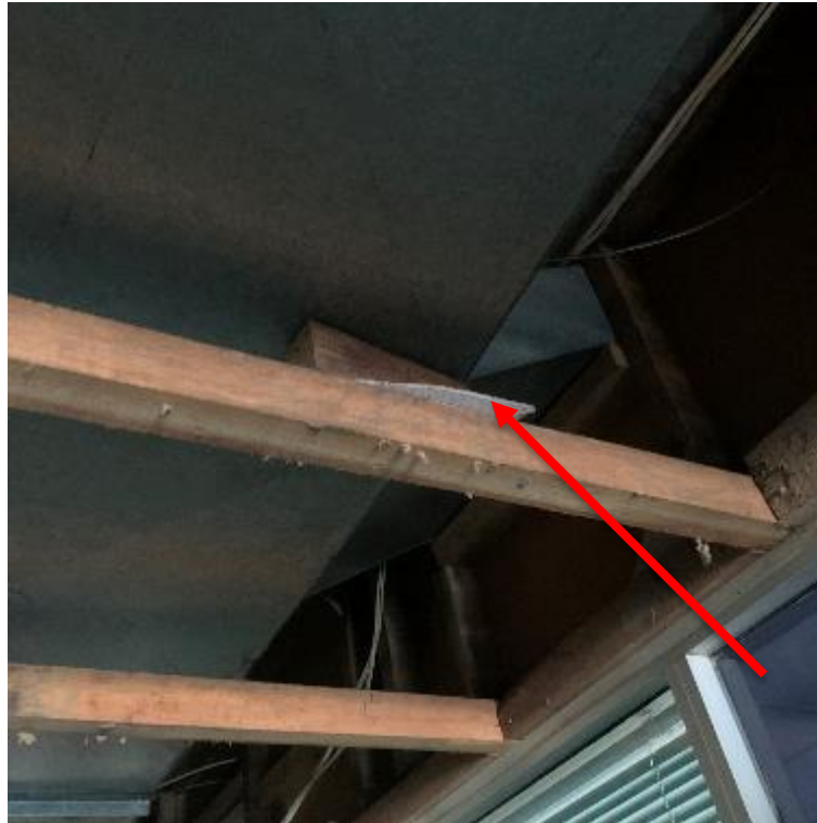
Image 3. Detail view of presumed asbestos cement sheet as packing material to air conditioning duct work within the Main Entry Corridor. This material should be removed as demolition works progress.
