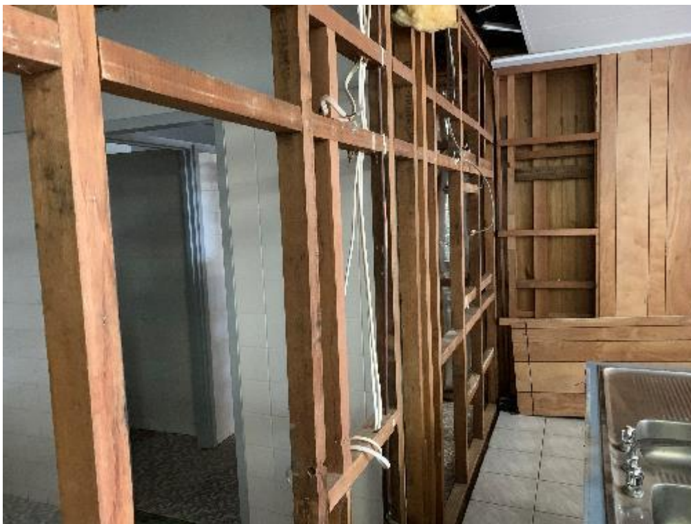
Image 4. View to the northeast wall of the Conference & Staff Room following the removal of asbestos cement sheeting.
