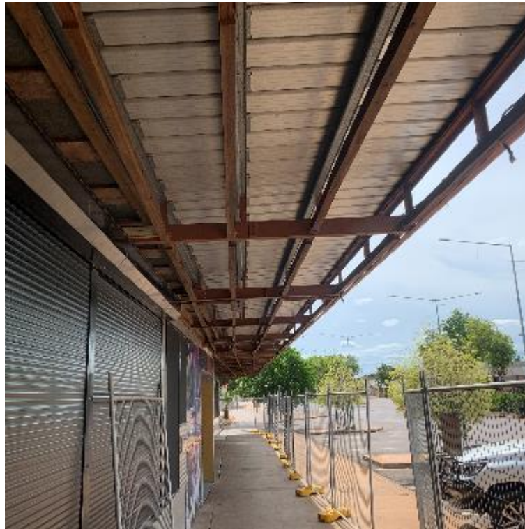
Image 1. View to the eaves and façade of the northeast elevation following the removal of asbestos cement sheeting.
